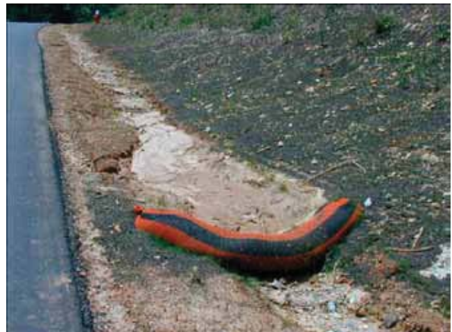
Figure 3 Compost filter sock check dam
